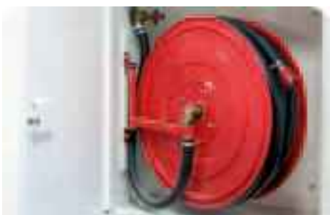
R.I.A. / Hose reel / Wandhydrant
